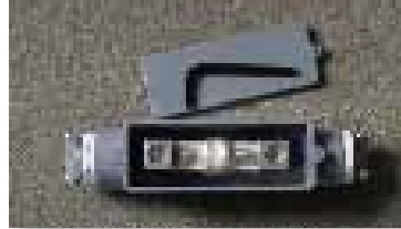
Class T fuse and cable terminals inside
