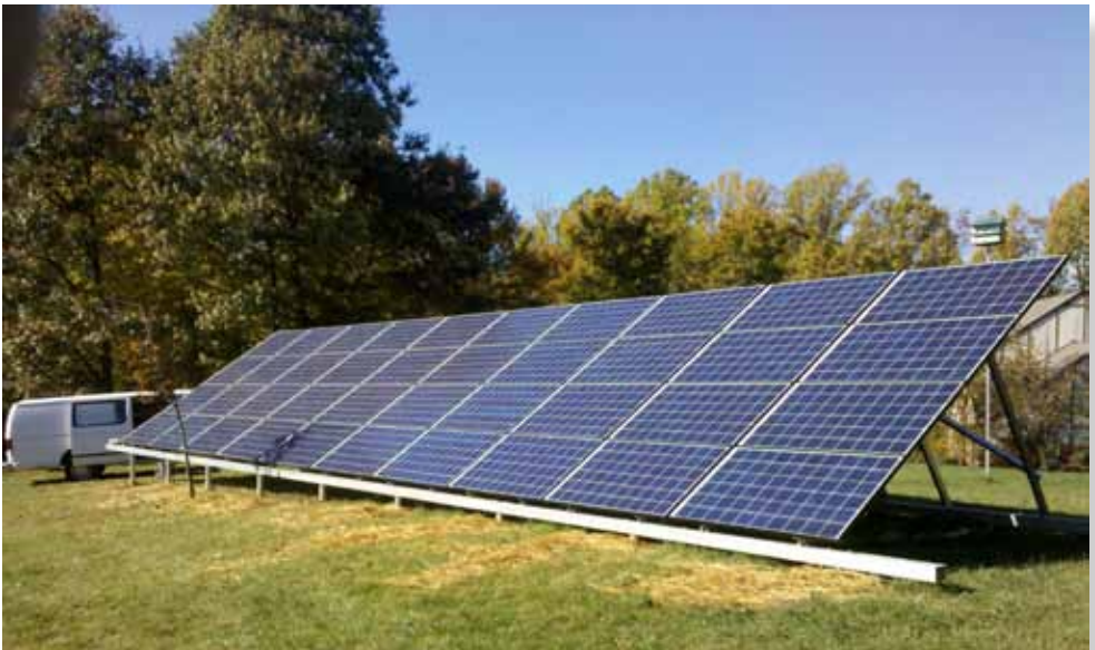
Photo courtesy of Joshua Galante of Altered Energy: SolarRacks ground mount system and REC modules
